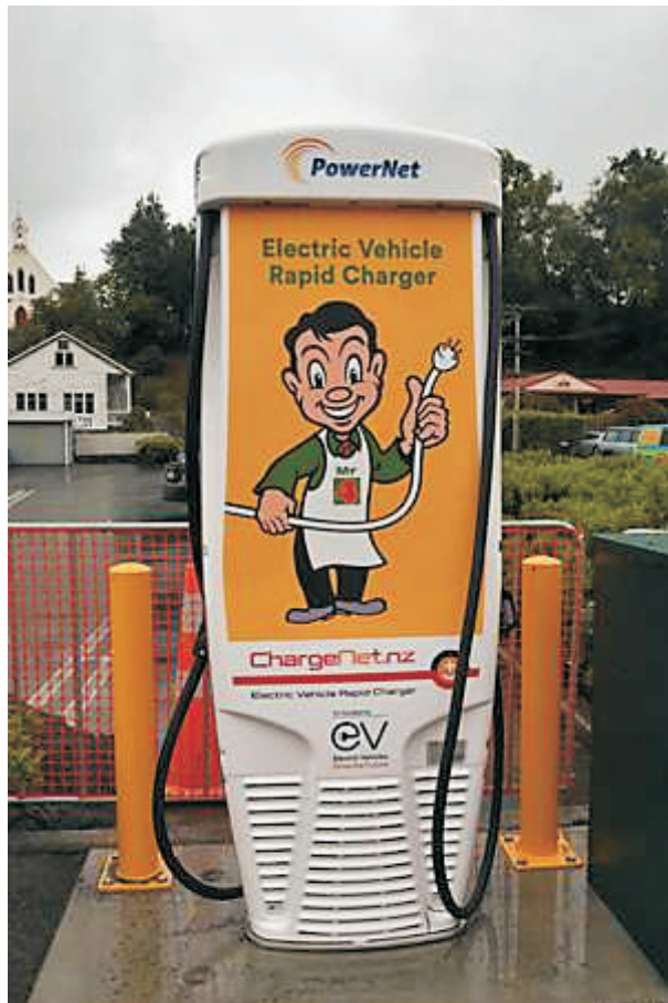
Electric power reaches Lawrence
