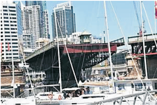
The bridge had come apart
